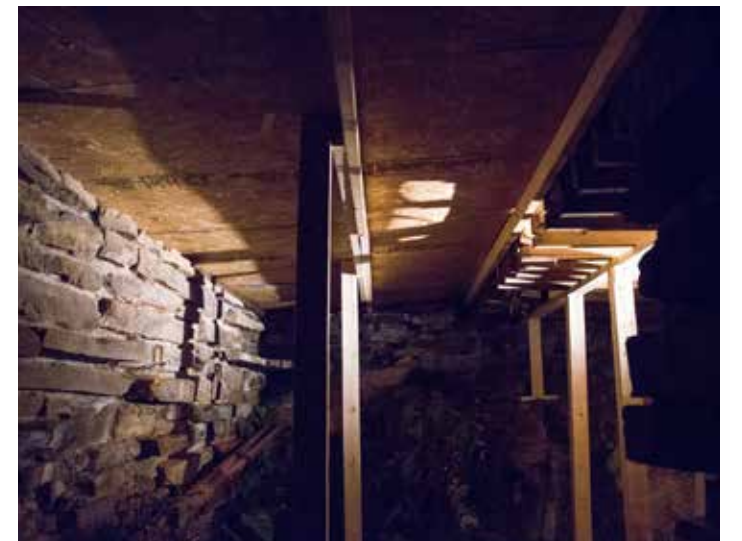
Middle, Fay Jones' home office studio on the home's ground level. Above, repairs to supports on the home's ground level. (Photos by Russell Cothren)
