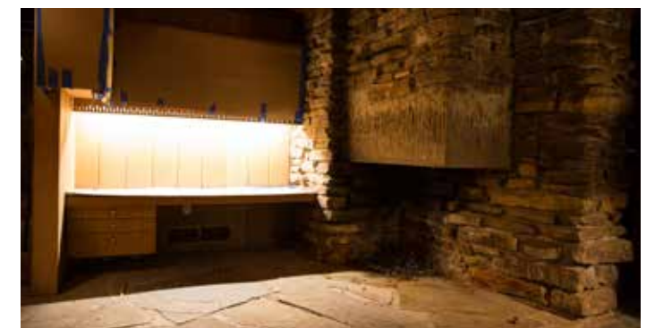
Clockwise from top left: Repairs made to the second floor living area include replacing the ceiling. A view from the front yard during restoration and repair work in fall 2017. A detail of the curved rock wall that runs along the driveway. The house number and another sculpture were part of Jones’ design. One of two built-in desks and the fireplace in the Jones daughters’ childhood bedroom. (All photos by Russell Cothren)
