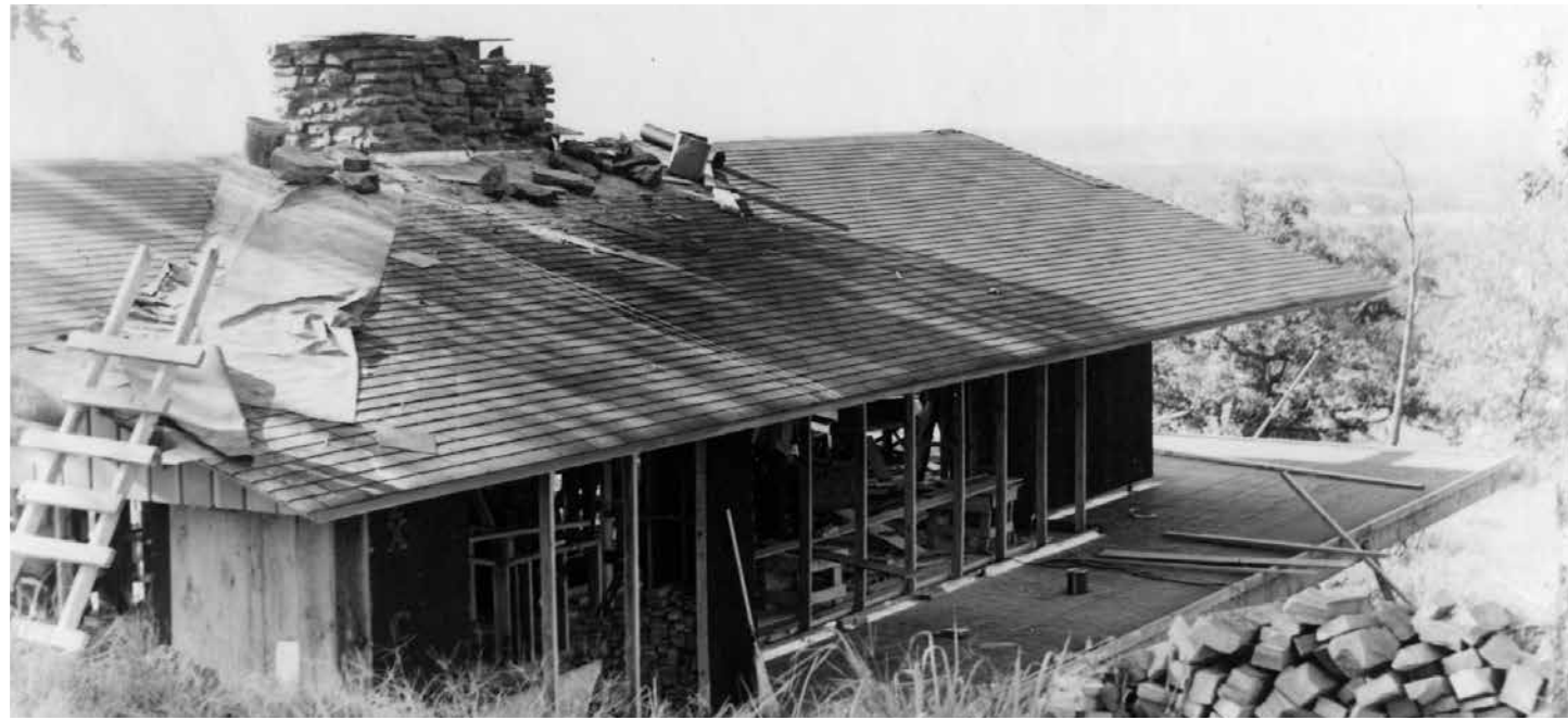
A view of the home under construction in the mid-1950s, looking northwest. (Image courtesy of Fay Jones Collection, Special Collections, University of Arkansas Libraries)
