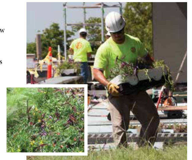
Workers with J.E. Allen Company install plants on the green roof of the Steven L. Anderson Design Center in June. Inset: A detail of the green roof plants.
